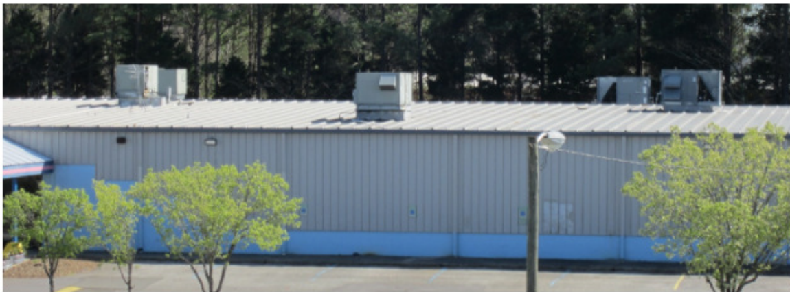
Skate Center RTUs (Photo taken from roof of Play Structure)
